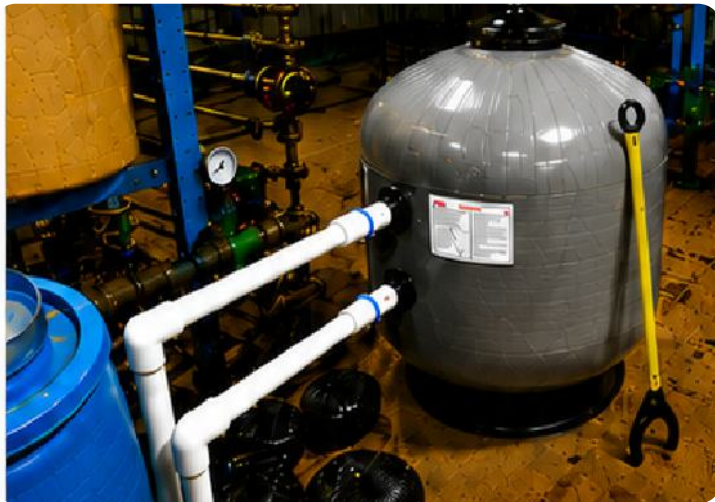
ProMoss® contact chamber installed during the field trial
