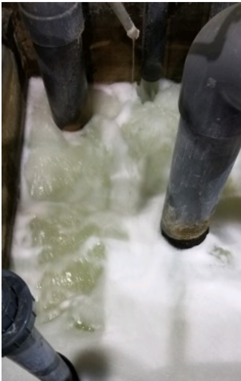
Picture taken of cooling tower sump on September 26th prior to ProMoss™ treatment
