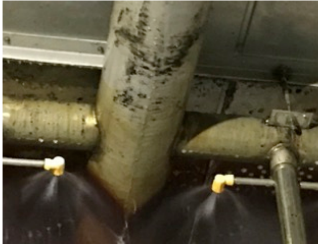
Spray Header Piping Before ProMoss™
